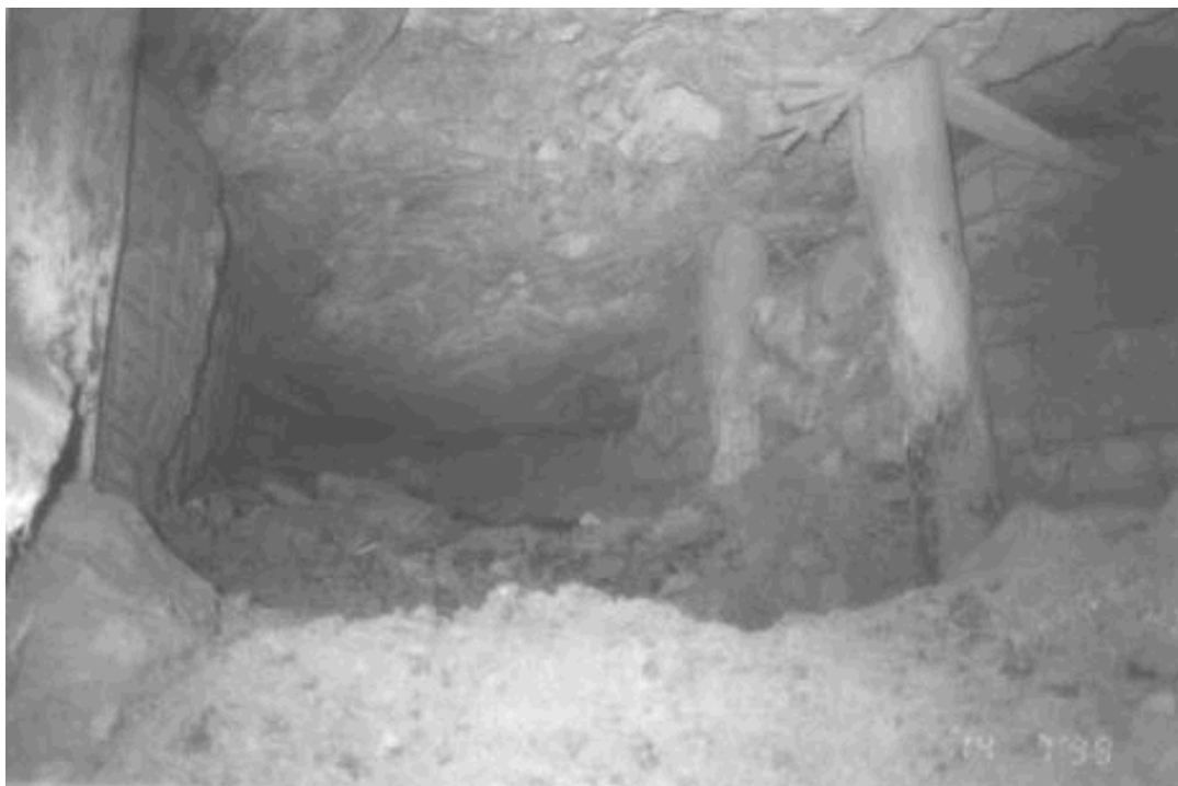
Figure 7-12. Example of variability of backfill placement at the Kopanang mine (South Africa) with a 1.5 m-wide gap left between backfill and the tunnel roof (from Squelch et al. 2001).
