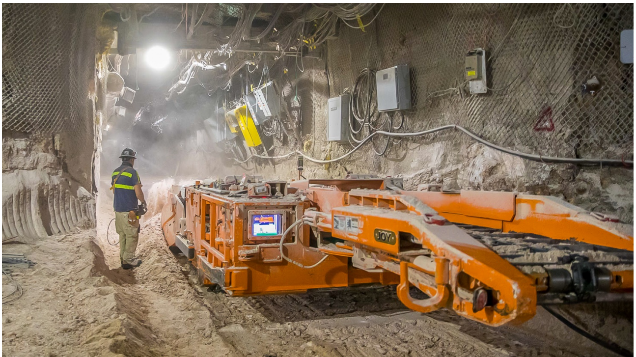
Figure 6.4-1. The WIPP GDF in New Mexico, USA, has been operational for over two decades. Image courtesy Nuclear Waste Partnership LLC (Carlsbad, USA).
